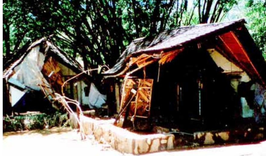
▲ One of the lodges at the Serena Mara which was damaged by the Mara river bursting its banks earlier this year.
